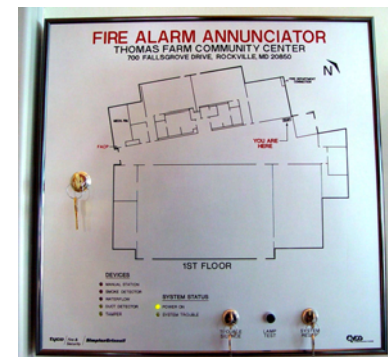
Thomas Farm Community Center Annunciator Panel
