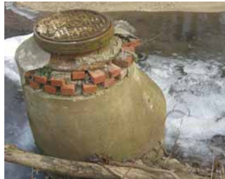
Deteriorated Sanitary Sewer Manhole to be Rehabilitated Through the Sewer Rehabilitation Program
