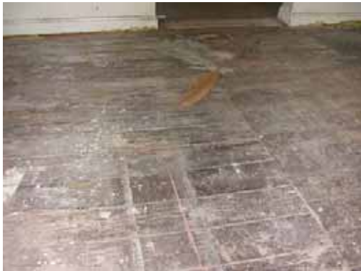
1 st floor yellow pine floor boards and possible "ghost" of dividing wall
