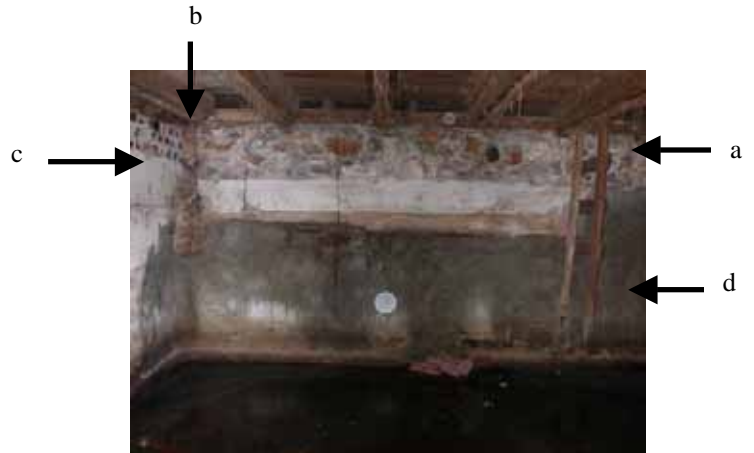
Cellar view showing original stone foundation (a), brick corner piers (b), brick perimeter foundation (c), concrete underpinning for cellar (d).
