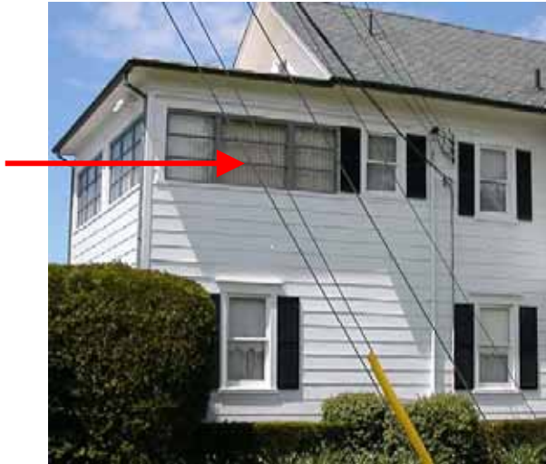
East façade of former porch. Upper windows on east (identified with arrow) to be replaced with unit of three.
