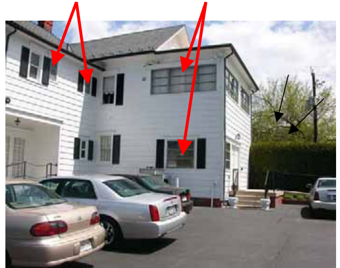
West façade of porch. Upper and lower windows on west (identified with arrows) to be replaced with unit of three. Two upper story bathroom windows on rear façade of main building to be replaced with singles.
