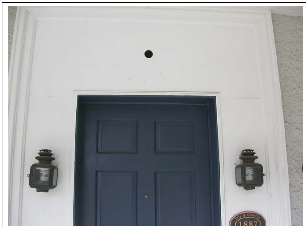
Plywood Door surround, with historic trim at the edges. Circle over the door is exploratory
