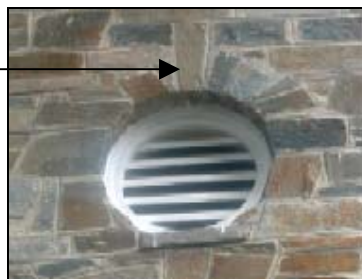
Circular louvered vent. Notice detail of stonework, upper right corner and projecting sill stone
