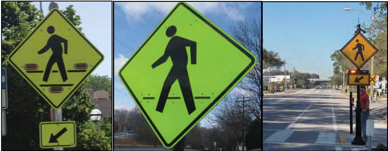
Figure 8 – LED Lights in Pedestrian Crossing Signs
