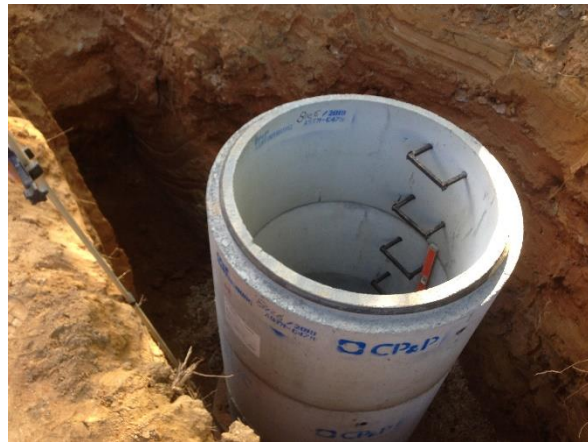
Underground Stormwater Piping
