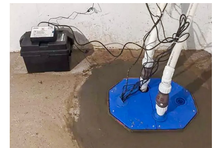
Battery backup for sump pump
