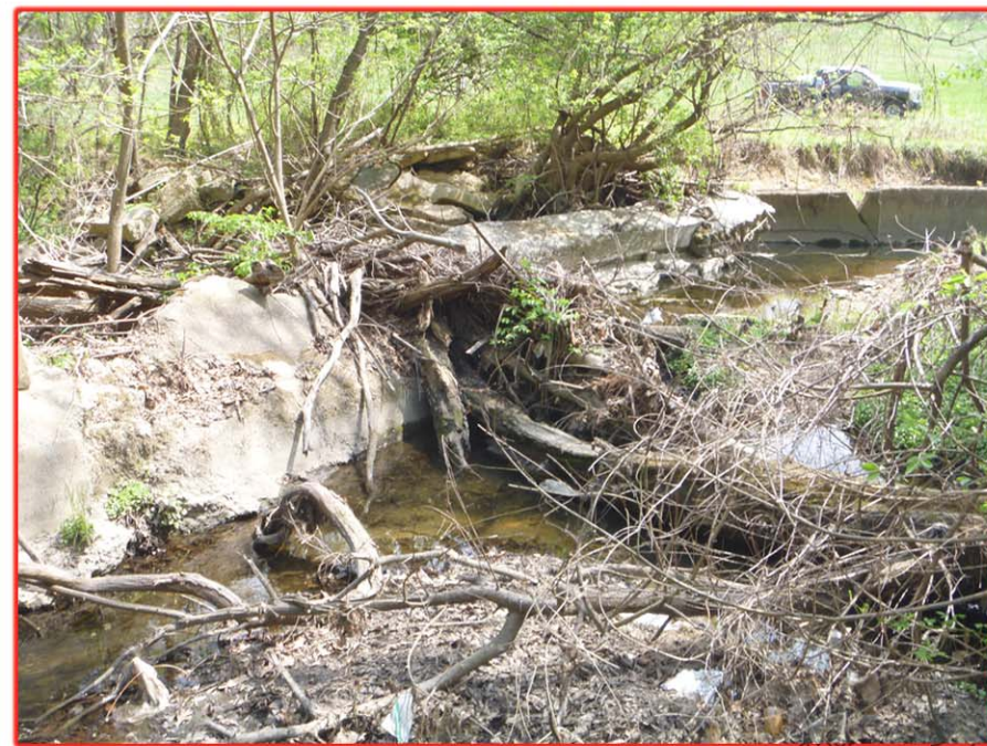
INSTREAM RUBBLE TO BE REMOVED
