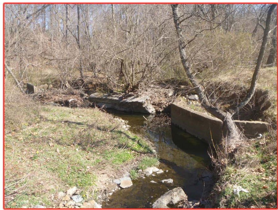
ERODED MEANDER BEND & CONCRETE RUBBLE TO BE REMOVED
