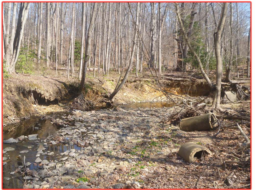
ERODING MEANDER BEND WITH UNDERCUT BANKS
