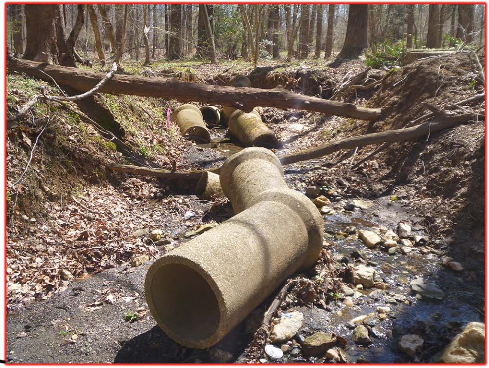
BROKEN STORMDRAIN OUTFALL
