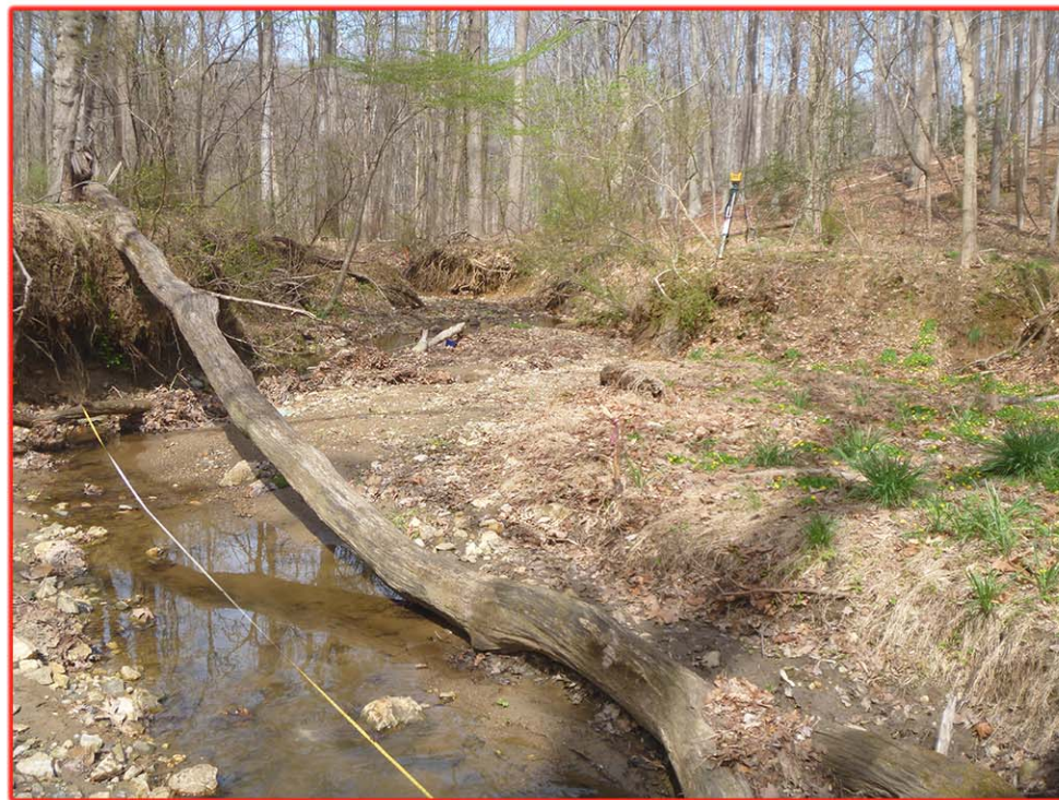
OVER-WIDENED CHANNEL WITH ERODED BANKS
