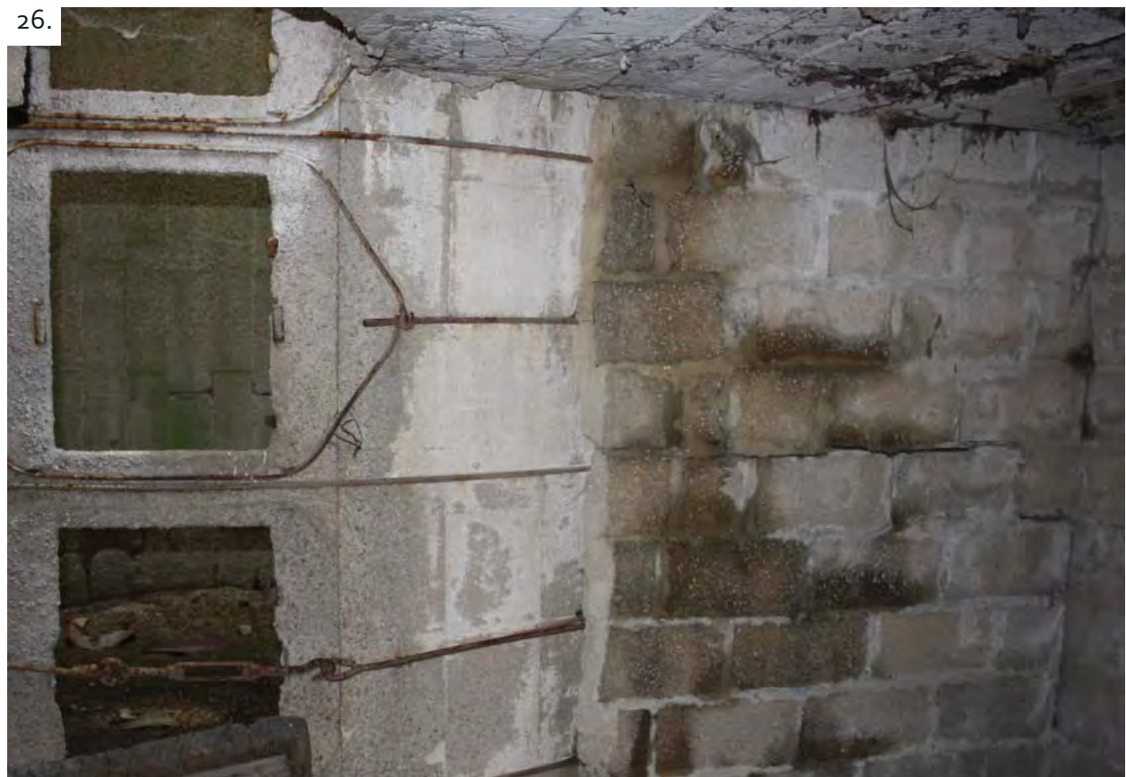
26. Connector 3 Significantly deteriorated and showing many signs of water damage.
