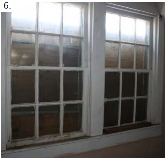
6. Stair Windows Sill in disrepair.
