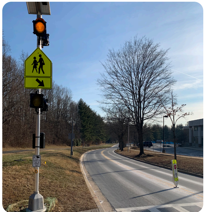
A pedestrian activated beacon on Wootton Parkway.
