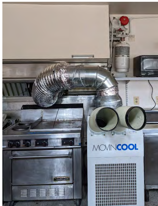
Figure 41: Kitchen Hood with ANSUL Fire Protection System and Temporary Cooling System
