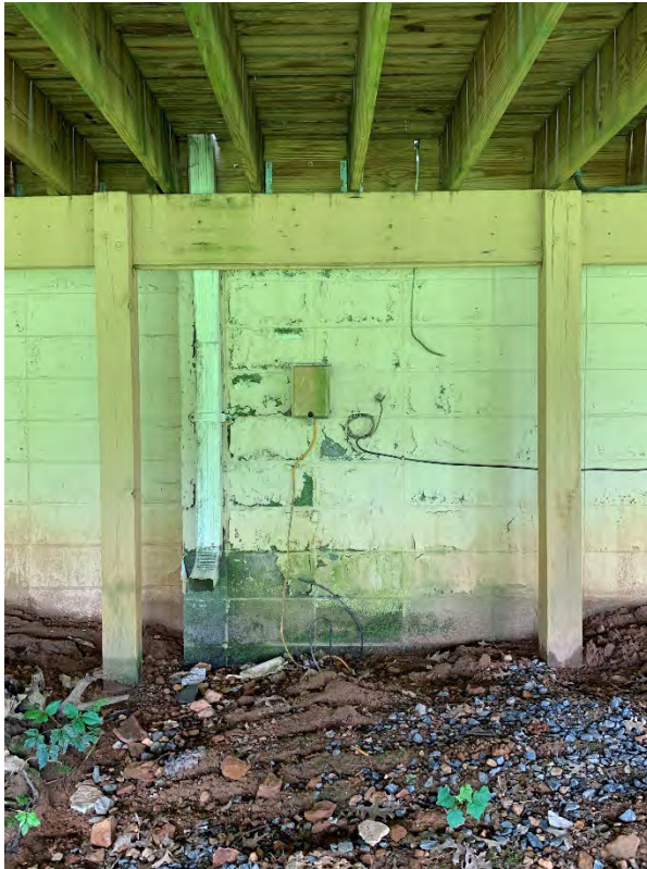
Figure 33: Masonry under Deck near Downspout
