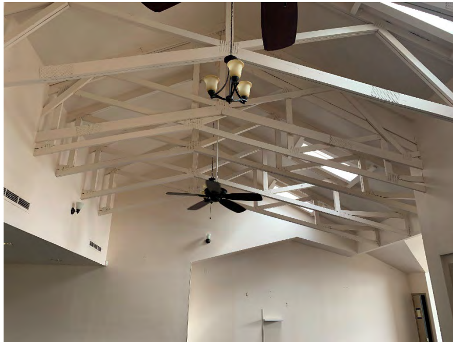
Figure 37: Typical Condition of Roof Trusses at Addition
