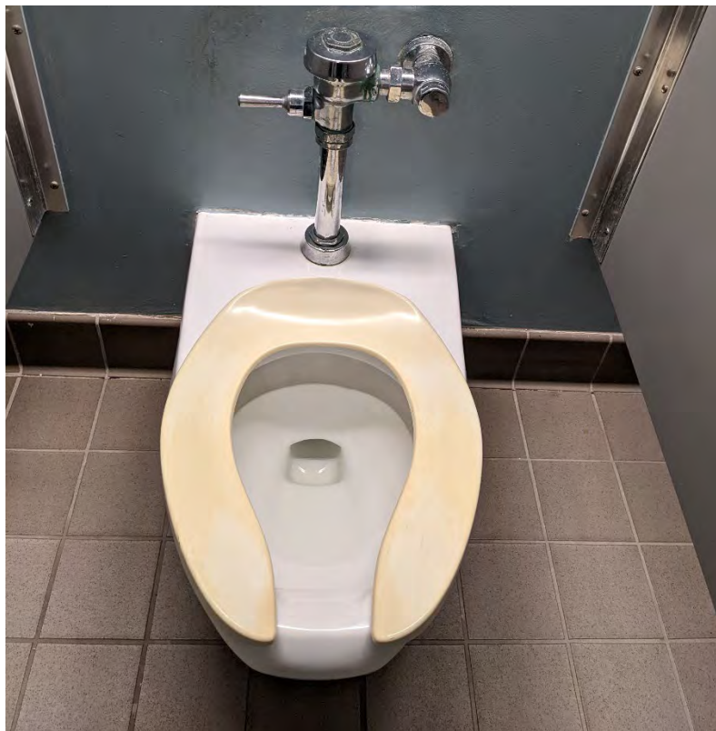
Figure 43: Typical Water Closet
