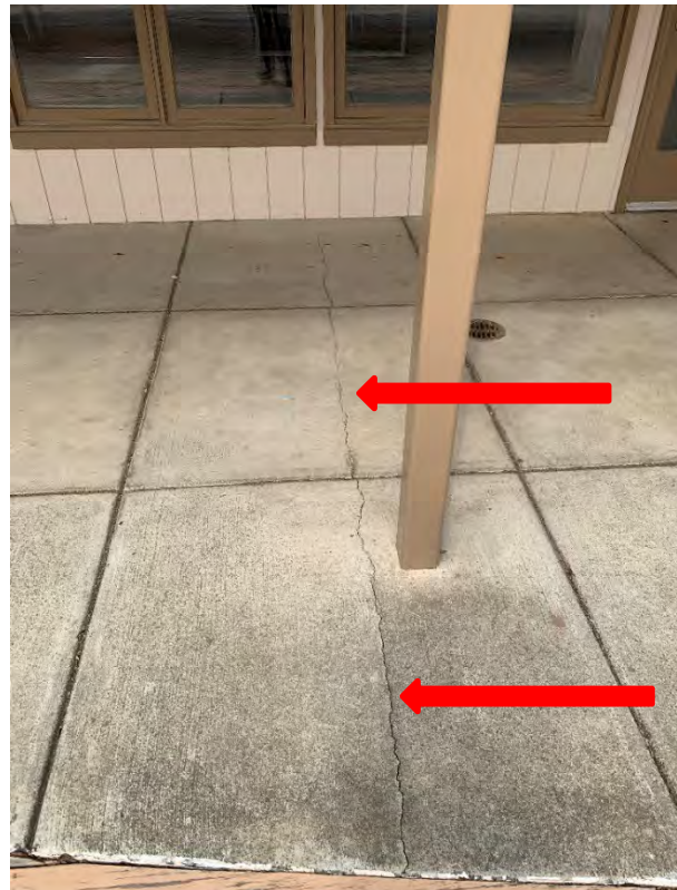
Figure 34: Crack at Terrace Slab
