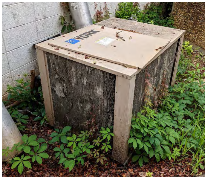
Figure 39: Dining Area Outdoor Unit
