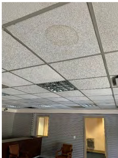
Fig. 24: ACT Ceiling Tile with Water Stains
