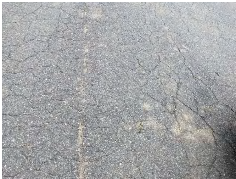
Figure 52: Alligator Cracks within Entrance Road
