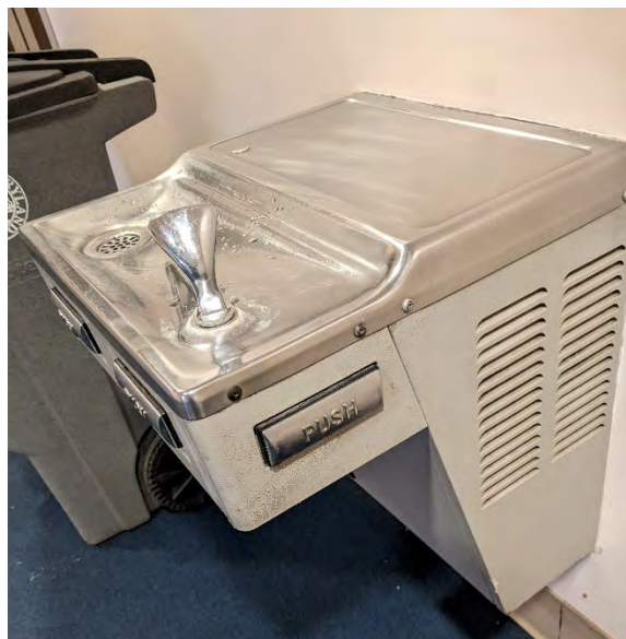
Figure 47: Electric Water Cooler
