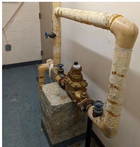
Figure 49: Domestic Water Insulation
