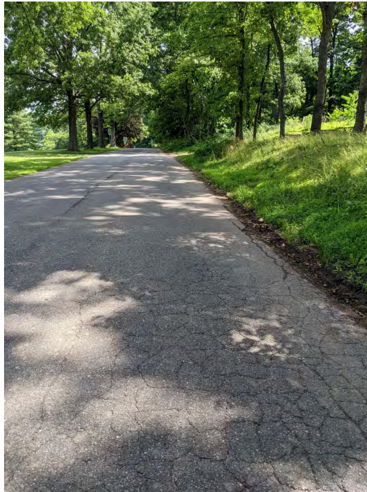
Figure 53: Alligator Cracking within Entrance Road
