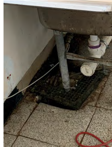
Fig. 32: Under Sink Condition
