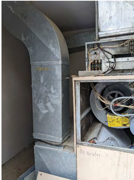
Figure 40: Dining Area Indoor Unit and Ductwork
