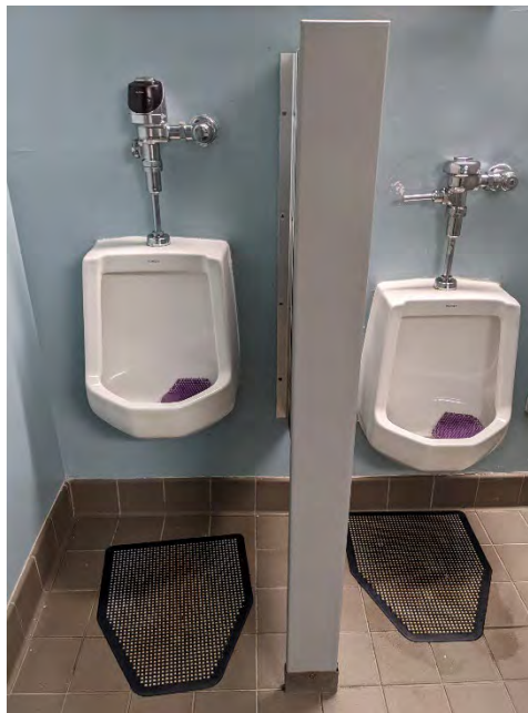
Figure 44: Urinals – One Sensor Flush Valve, One Manual Flush Valve
