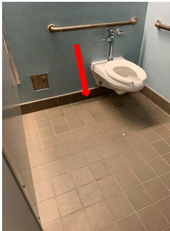
Figure 36: Separation of Floor and Wall Finishes at Men's Bathroom
