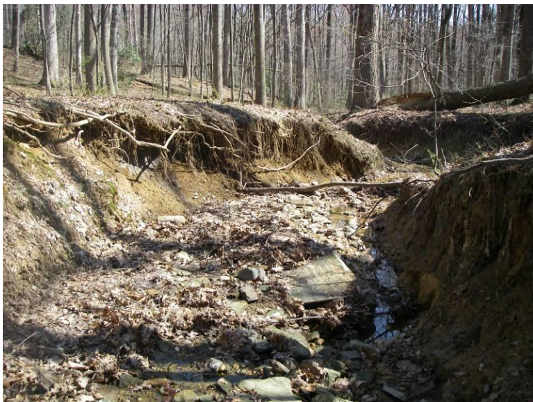
FIGURE 15: SEVERE BANK EROSION (REACH BOG-005)
