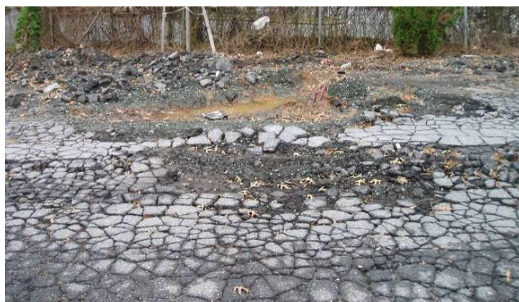
FIGURE 48: PARKING LOT IN NEED OF REPLACEMENT (H-101).
