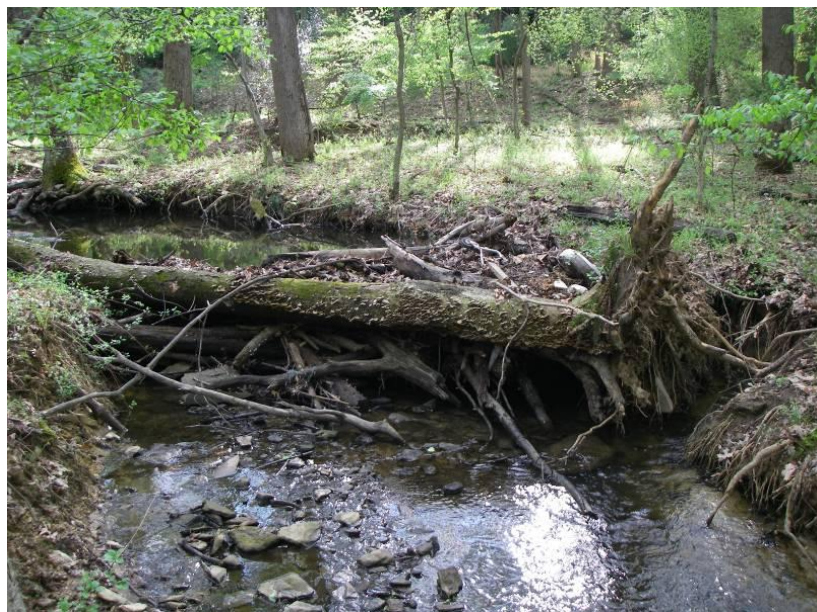
FIGURE 39: DEBRIS JAM CONTRIBUTING TO EROSION (REACH OFC-015)
