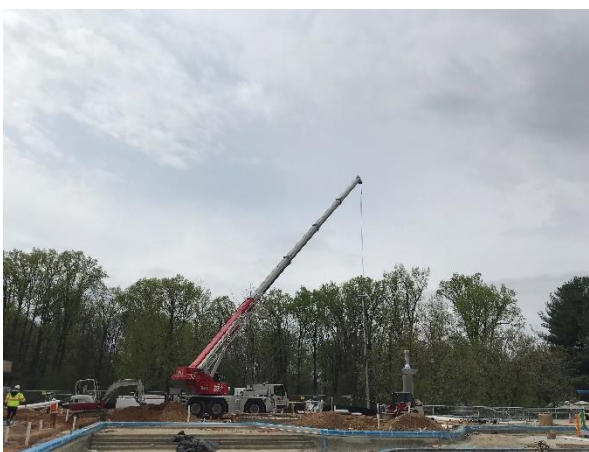
Light Pole Placement
