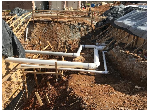
Water Slide Piping
