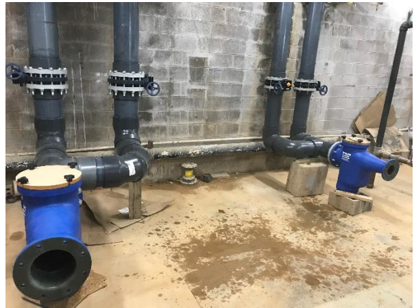
Filtration System Components
