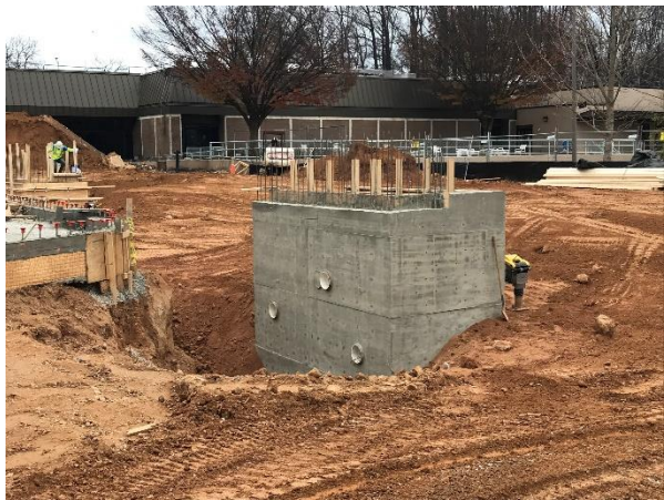
Activity Pool Surge Tank
