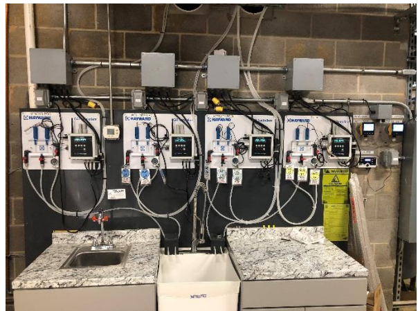
Pool Chemical Controllers
