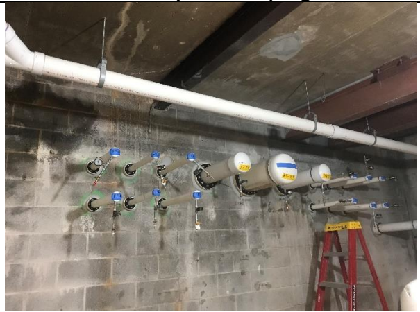
Pool Piping Into Filter Room
