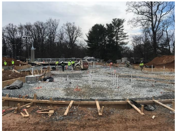
Activity Pool Piping
