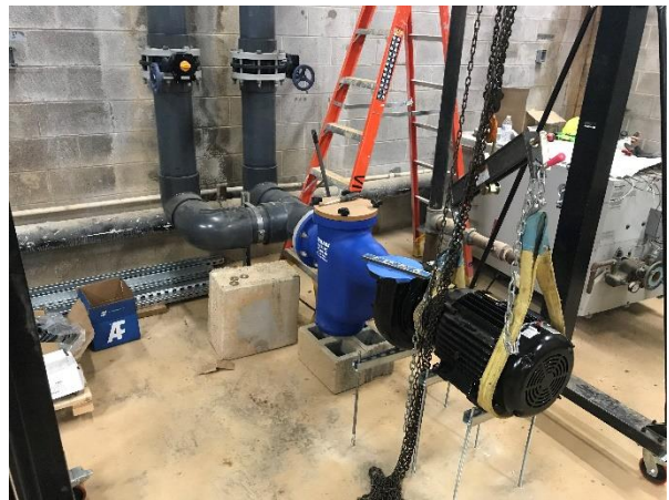
Filtration System Components
