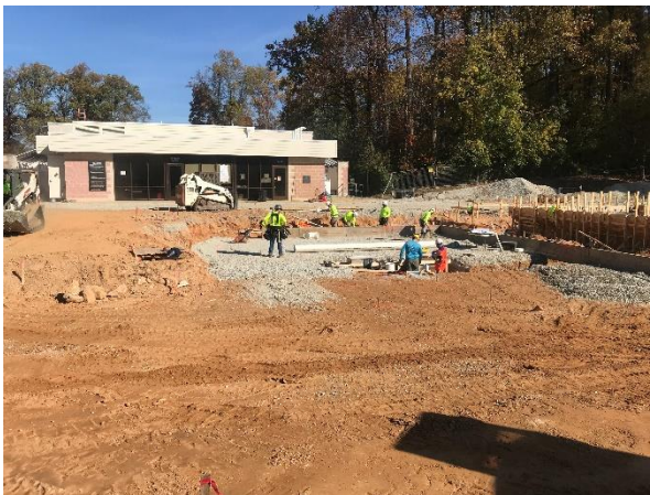
Activity Pool Piping
