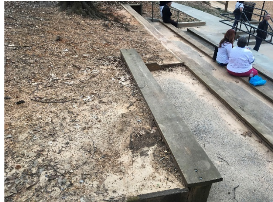
Erosion & Sedimentation at Northern Baseball Fields
