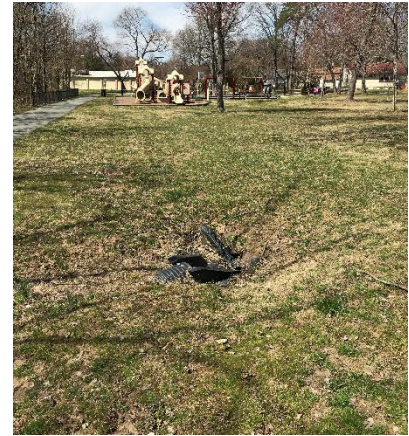
Exposed Drainage Inlet / Outfall
