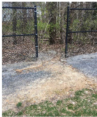
Drainage/Erosion at Ballfields
