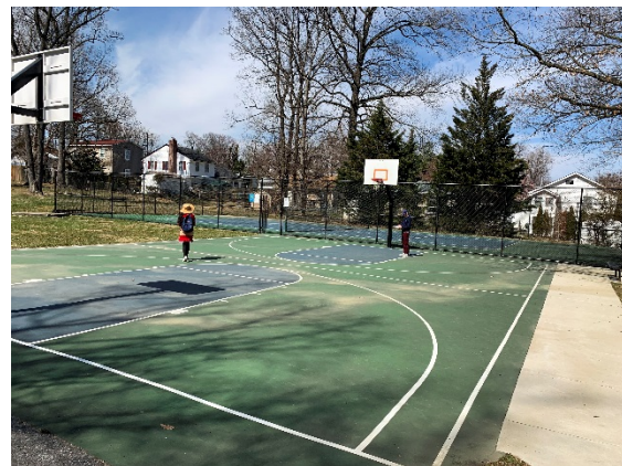
Soil Washes onto Hardcourt Surface
