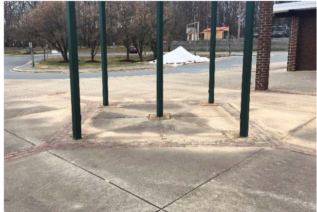
Sedimentation Issue at the Plaza
