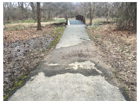
Flooding and Sedimentation over Trail
