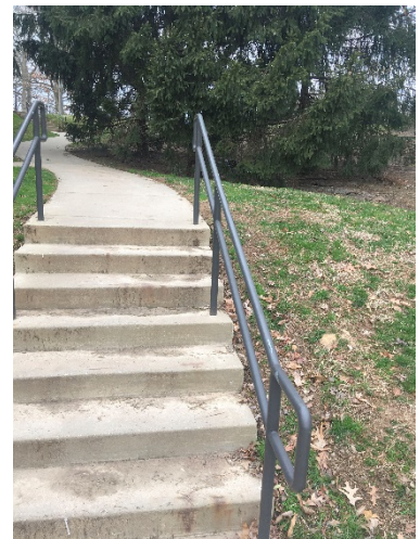
Drainage Issue near the Civic Center
