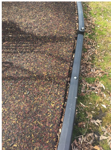
Edging Separating from Playground Surface
