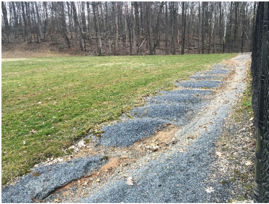
Severe Erosion at Southern Baseball Field
