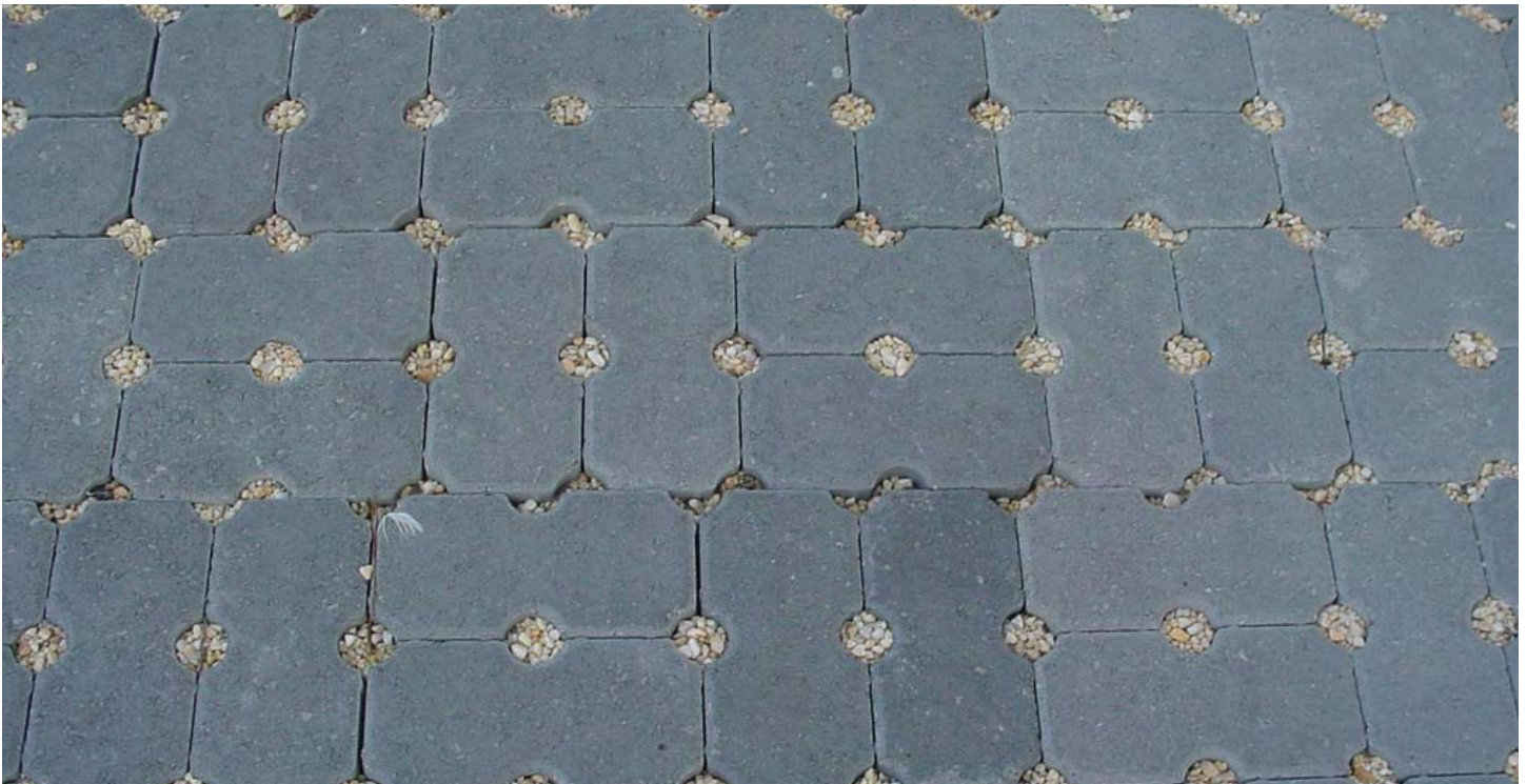
Poorly aligned pavers
