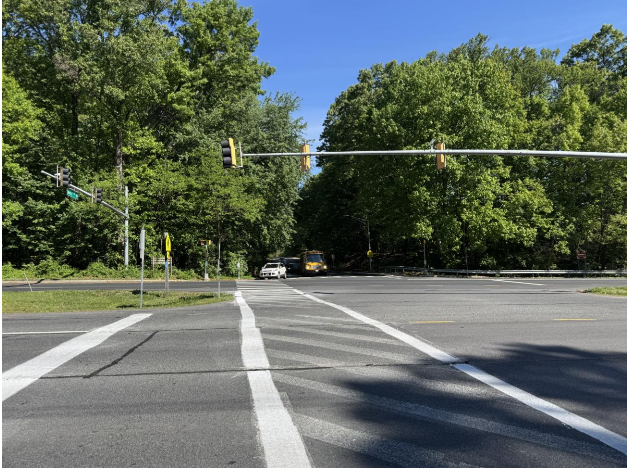
Figure 118. Long west leg pedestrian crosswalk deteriorated and lacking high visibility design on south side #18 - Norbeck Road (MD 28) & Avery Road
