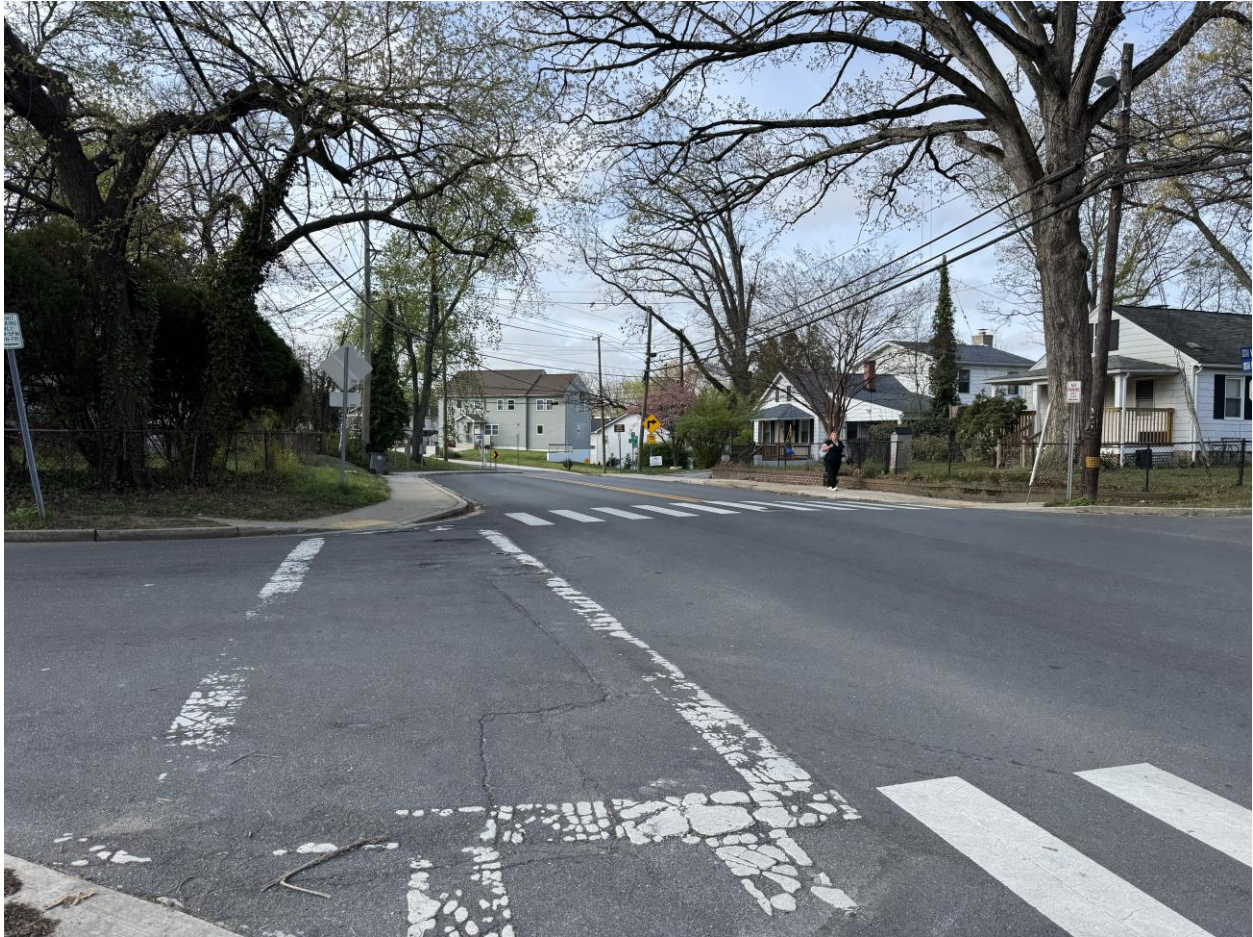
Figure 64. Faded crosswalk marking with missing transverse white marking across westbound approach of Woodland Road at Intersection #10 – Woodland Road & N. Horners Lane
