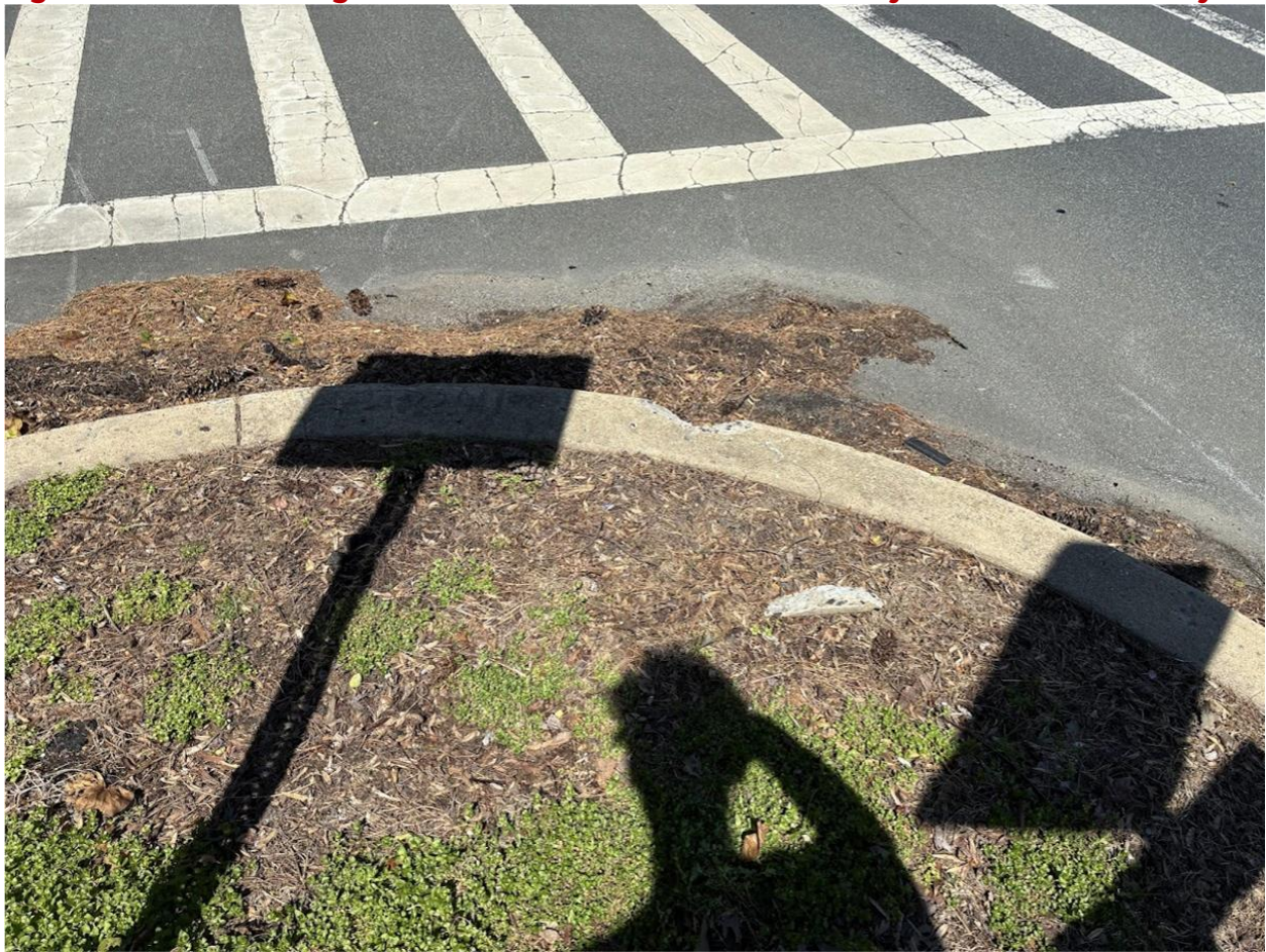
Figure 8: Median Damage at Intersection #1 – Wootton Parkway & Pasture Brook Way
