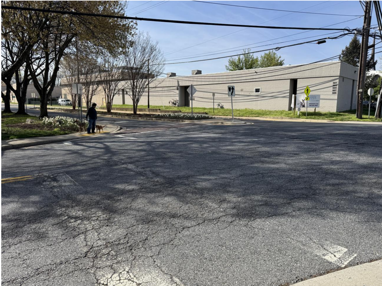
Figure 58. Faded crosswalks and stop bar near the stop sign at Baltimore Road at Intersection #9 – Baltimore Road & S. Stonestreet Avenue
