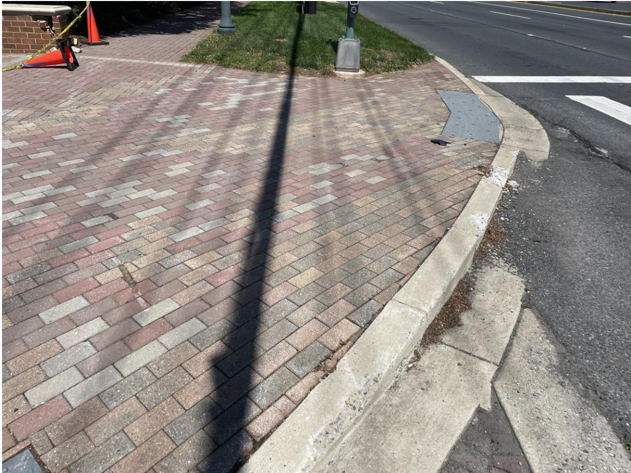
Figure 87. Damaged curb ramps and brick crosswalk on east leg #13 - Frederick Road (MD 355) & Watkins Pond Boulevard
