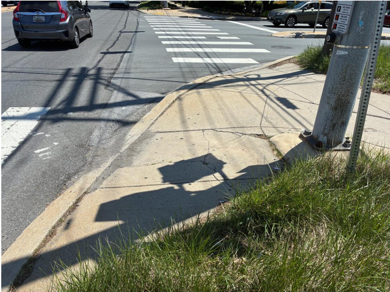
Figure 132. Missing ADA-compliant curb ramps at Intersection #20 - Rockville Pike (MD 355) & Congressional Lane
