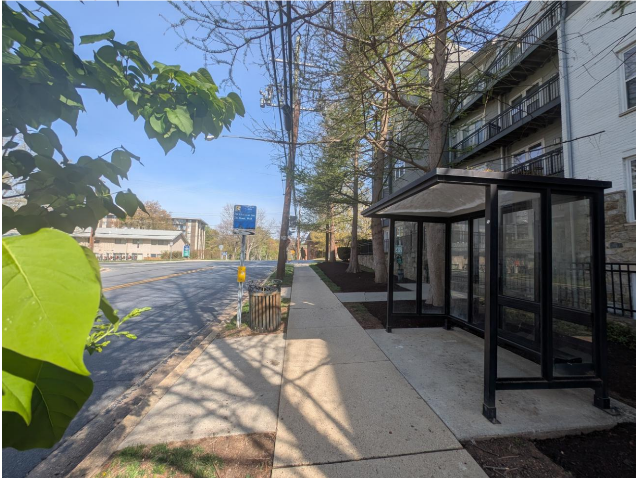
Figure 48. Bus stop at the southeast corner of the intersection is missing ADA-compliant amenities, bus pad, and parking regulation signage at Intersection #7 – E. Jefferson Street & Congressional Lane
