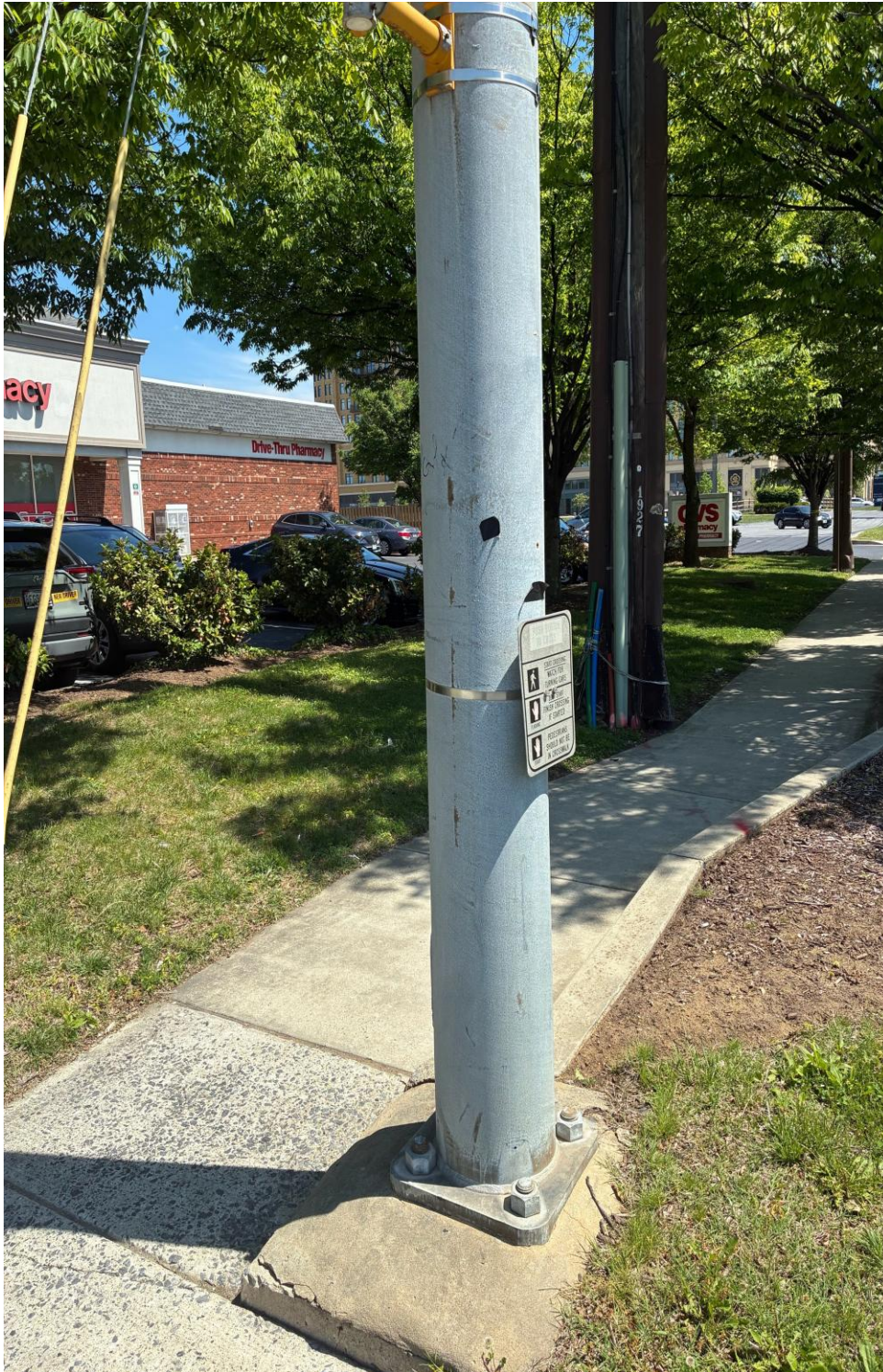
Figure 131. Missing pedestrian push button at Intersection #20 - Rockville Pike (MD 355) & Congressional Lane
