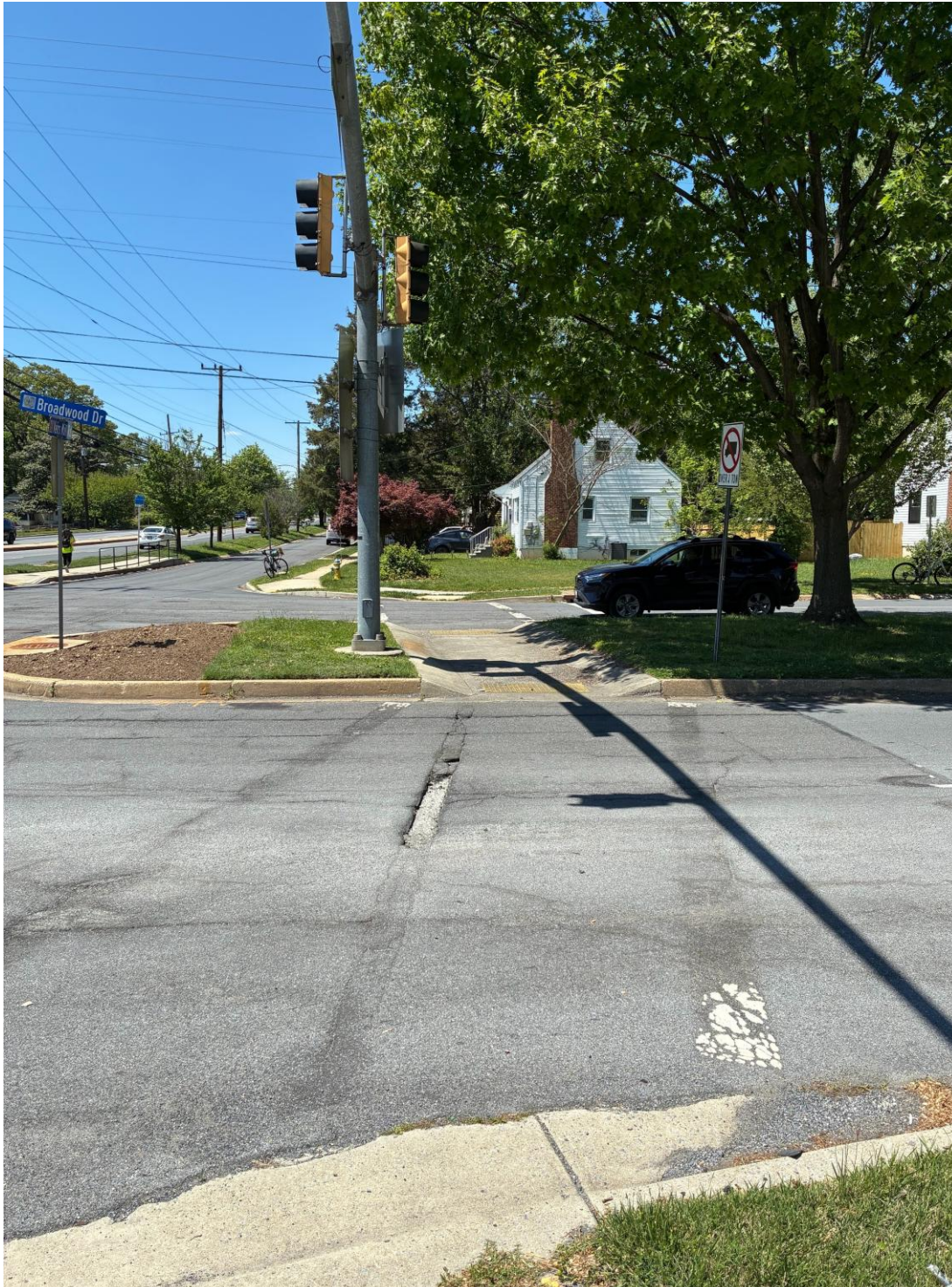
Figure 99. No pedestrian signal heads or push buttons on the southbound approach at Intersection #15 - Veirs Mill Road (MD 586) & Broadwood Drive
