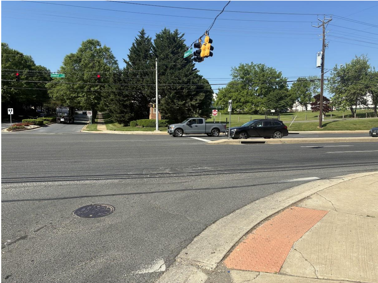
Figure 158. Missing crosswalk on the southbound approach at Intersection #24 - Frederick Road (MD 355) & Ridgemont Avenue
