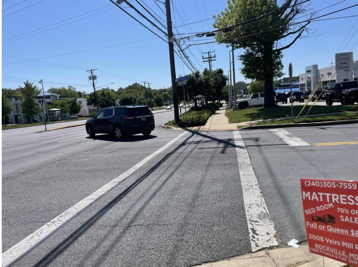
Figure 192. Deteriorated pavement markings on the west leg pedestrian crosswalk and lacking high-visibility design at intersection #30 - Rockville Pike (MD 355) & Mt. Vernon Place
