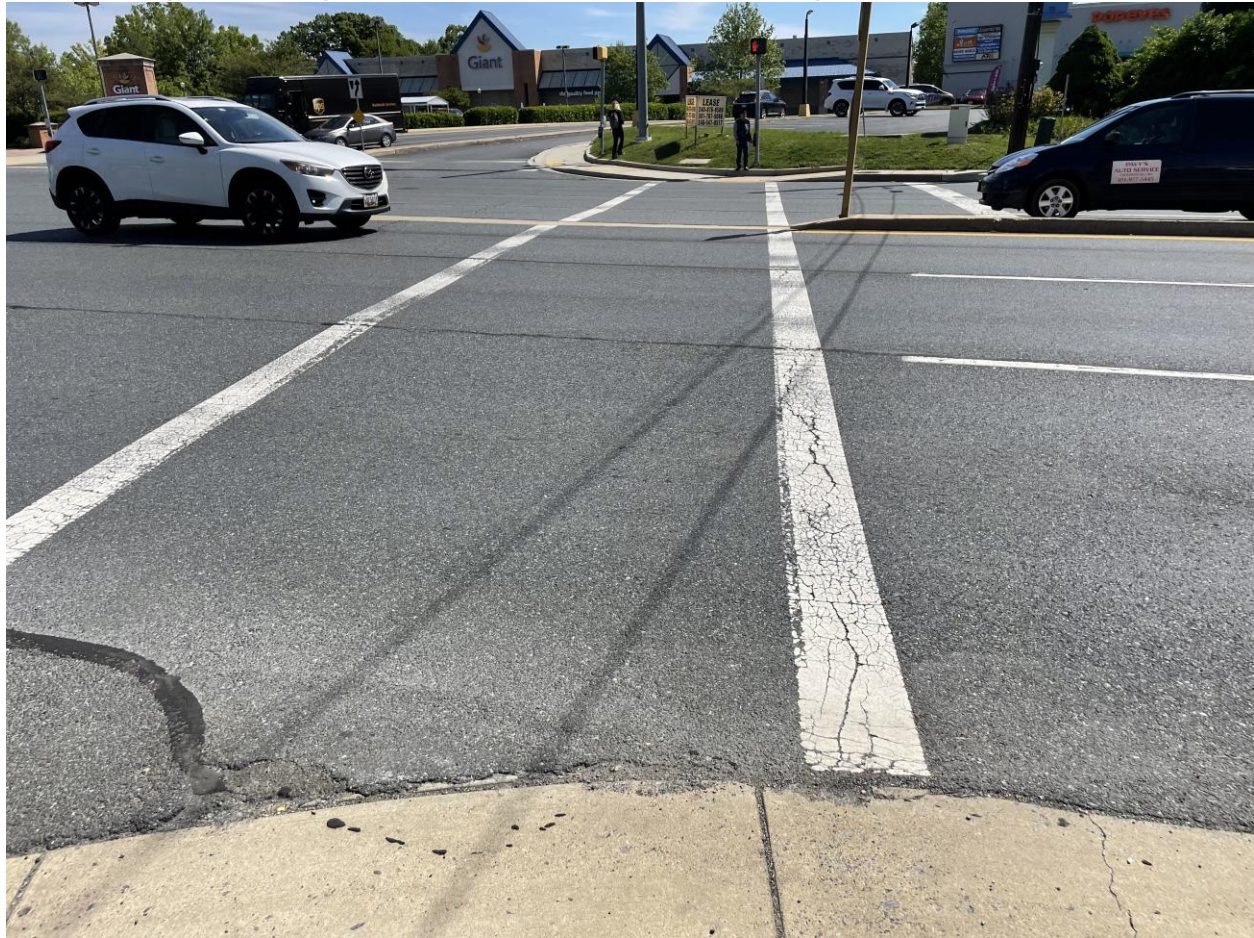
Figure 79. Long crosswalk frequently used by pedestrians lacking high visibility pattern on south leg #12 - Hungerford Drive (MD 355) & N. Washington Street
