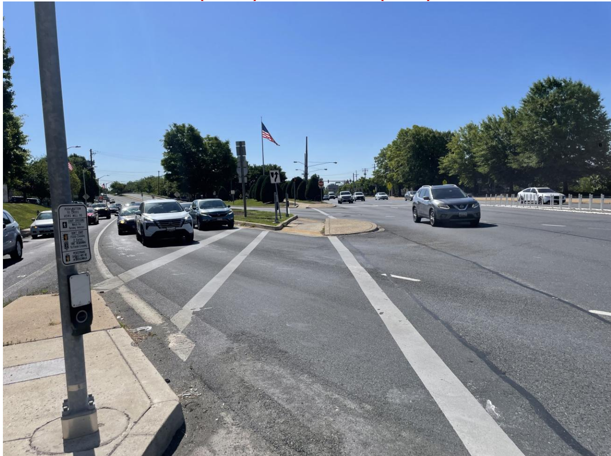
Figure 138. Long pedestrian crosswalk along the west leg with faded pavement markings, lacking high visibility design, and crosswalk signals difficult to see across long distance #21 - Rockville Pike (MD 355) & Veirs Mill Road (MD 28)
