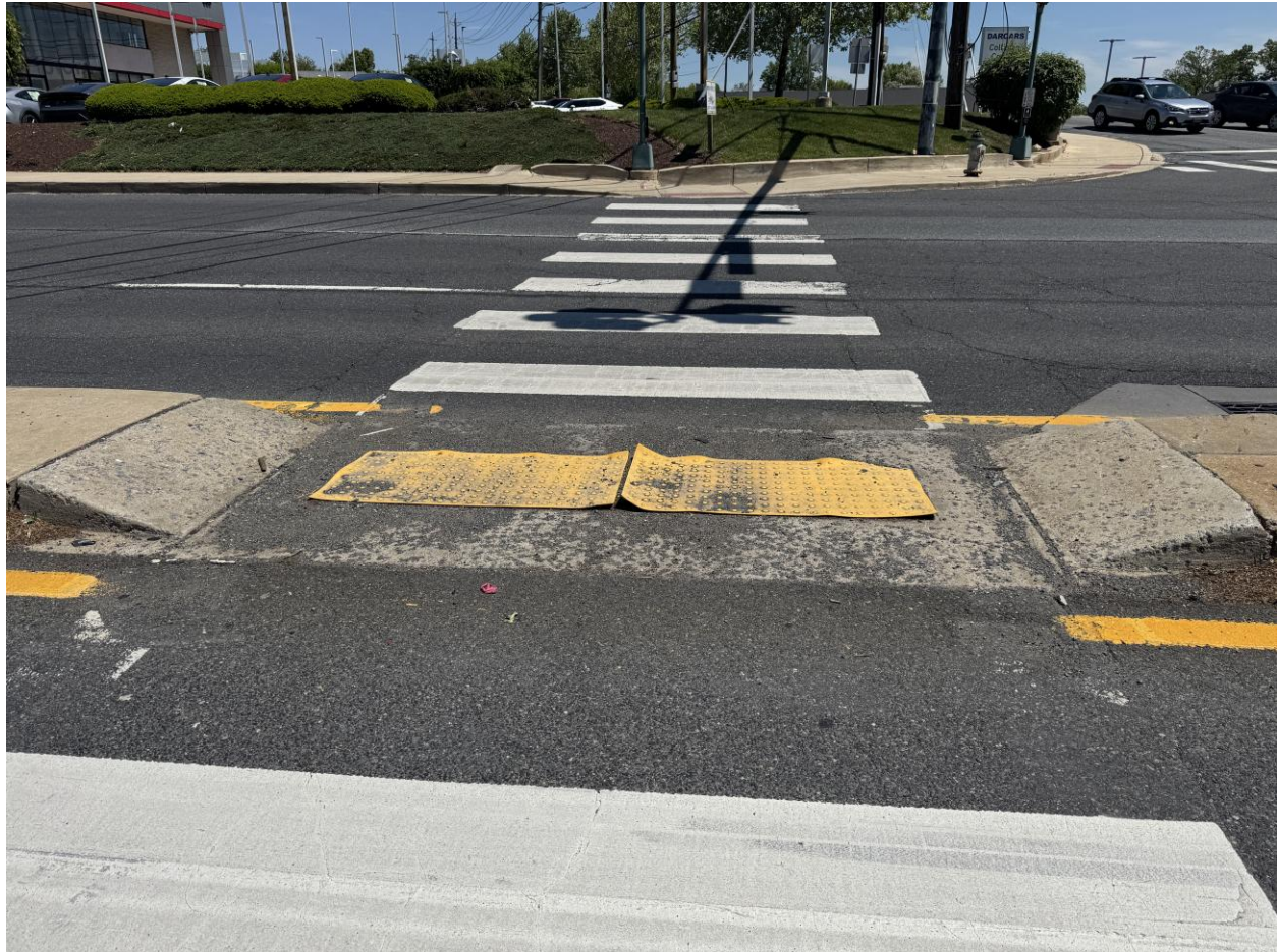
Figure 86. Deteriorated crosswalk pavement markings and detectable warning surfaces #13 - Frederick Road (MD 355) & Watkins Pond Boulevard
