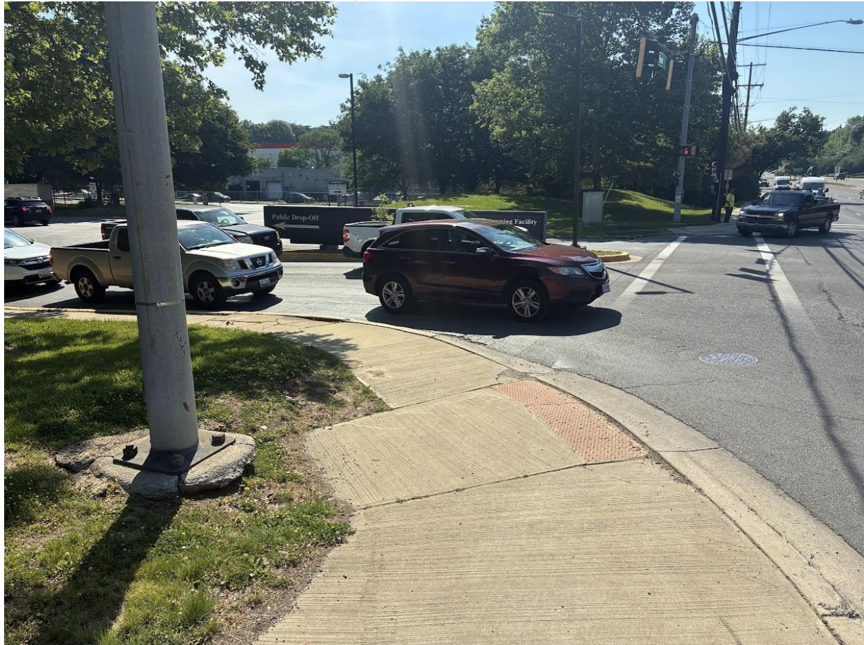
Figure 157. Missing pedestrian push buttons on the westbound approach at Intersection #24 - Frederick Road (MD 355) & Ridgemont Avenue
