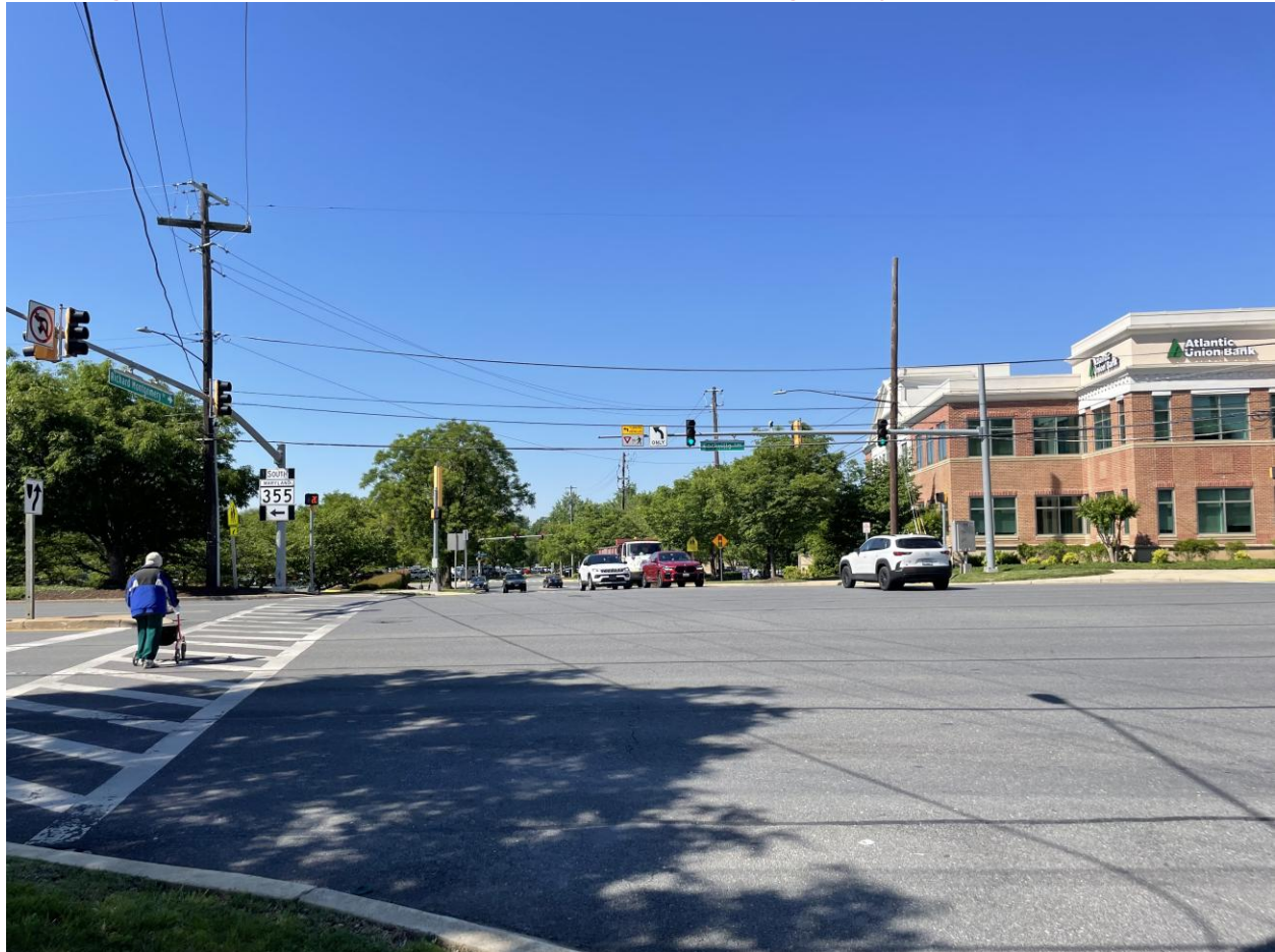
Figure 150. Long pedestrian crosswalks on north and south legs with faded pavement markings #23 - Rockville Pike (MD 355) & Richard Montgomery Street
