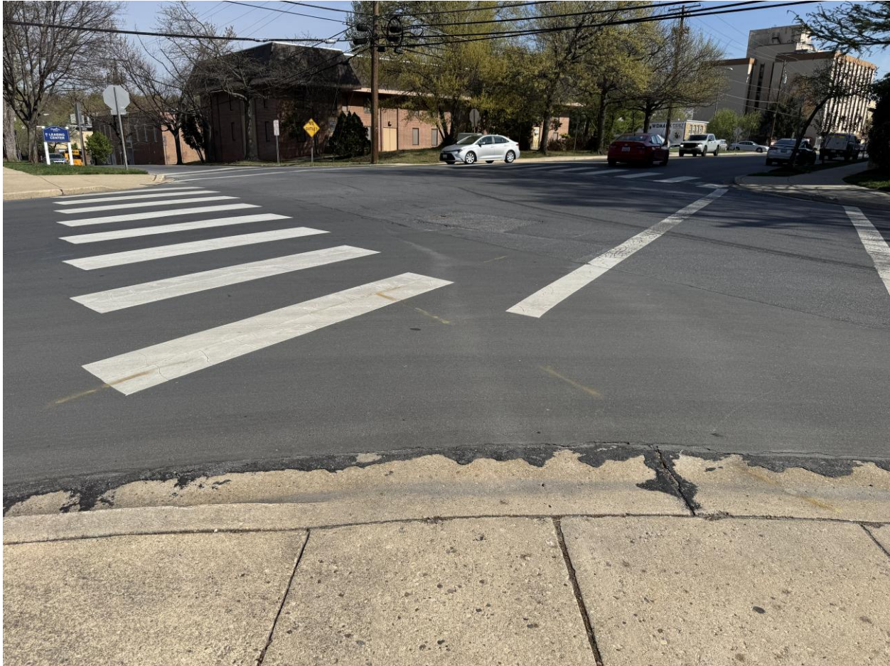
Figure 46. Crosswalks missing ADA-compliant detectable warning surfaces, horizontal and transverse solid white line at Intersection #7 – E. Jefferson Street & Congressional Lane
