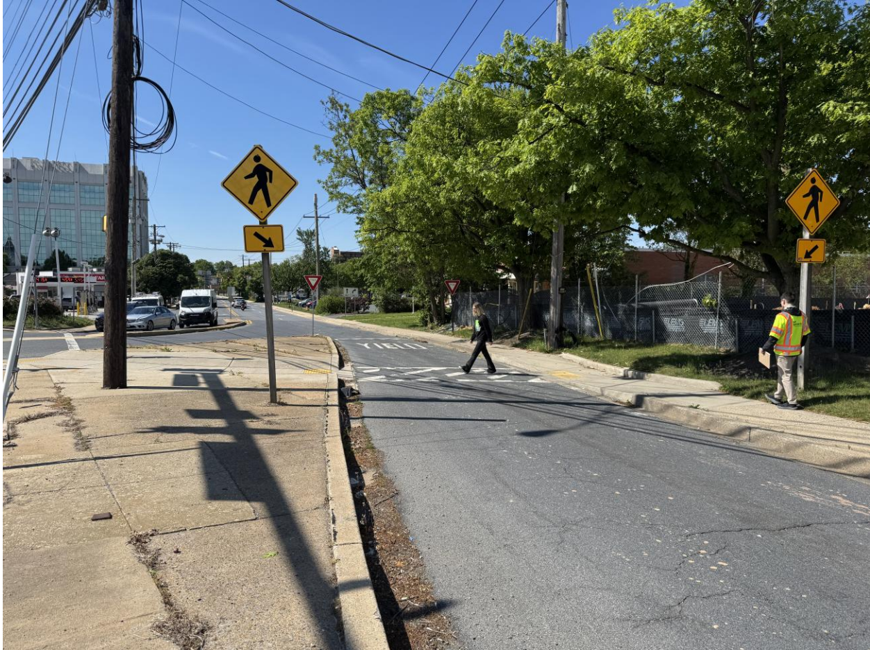
Figure 78. Faded high visibility crosswalk and pedestrian crossing signs on southbound approach slip lane #12 - Hungerford Drive (MD 355) & N. Washington Street
